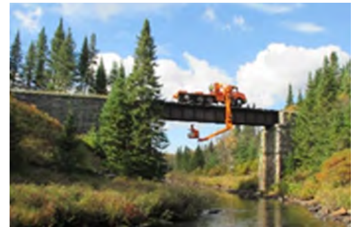
Location: Jefferson, Lewis and St. Lawrence Counties, NY Owner: MA&N Railroad/ St. Lawrence County IDA Completion: 2018
