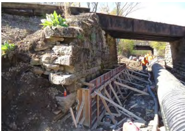
Two of the bridges required long-term diversion of a designated trout stream in order to complete the work.
