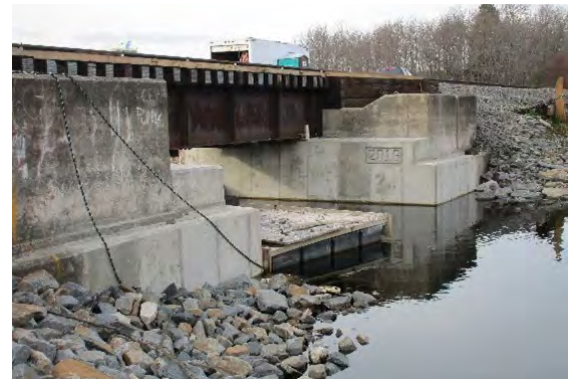
The DL Bridge 113.52 over Larsen Lake project involved underwater repair work performed by skilled divers.
