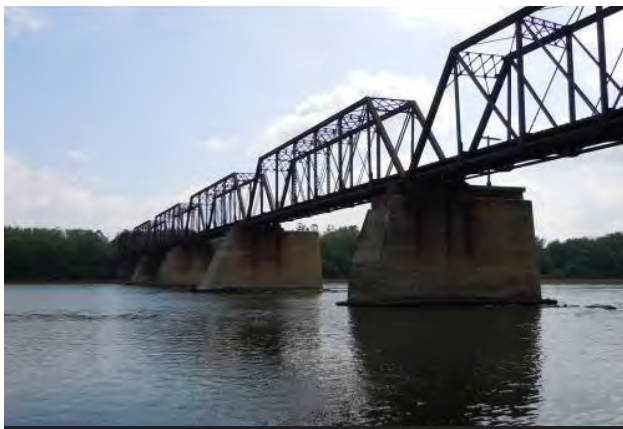
Pier and bearing stone repairs were performed on the 8-span, 1,170-foot-long Bridge 143.19.
