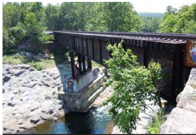
Work at Bridge 8.45 consisted of bearing repair, repointing the masonry piers and abutments, and repairs to deteriorated stones at one wingwall.
