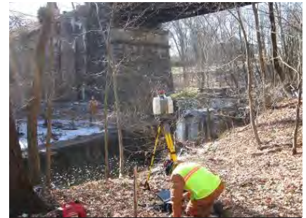
Laser scanning was used at SEPTA Bridge 20.25 to capture detailed information for tall stone abutments that could not be accomplished otherwise.
