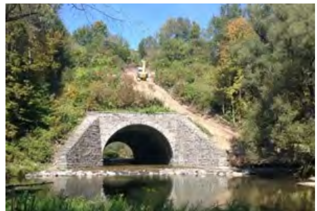
Geosynthetic Reinforced Soil Slope washout repairs underway at the 80'-tall embankment fill at Bridge 16.30.
