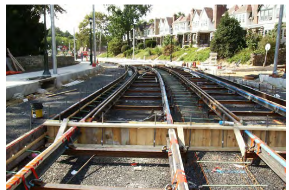
Construction inspection for special trackwork for the reconstruction of Germantown Avenue outside of Philadelphia.
