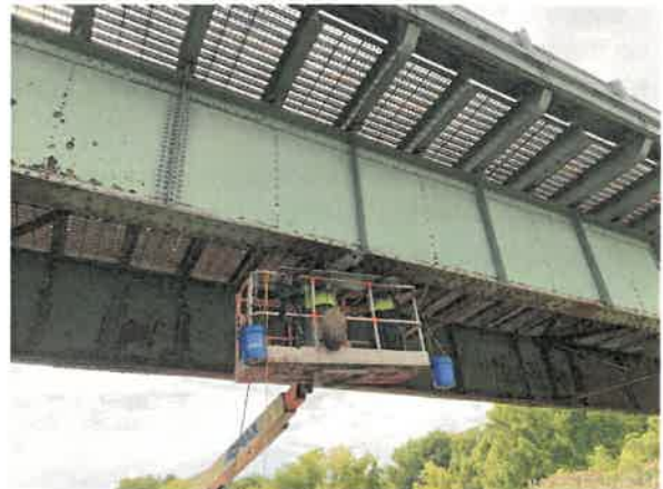
FIGURE 4: Parsons assisted the Authority in the prompt repair of conditions discovered as part of the 2023 SILO Inspection.
