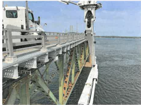
FIGURE 5: Parsons bridge inspection team accessing the approach truss of the Ogdensburg-Prescott International Bridge for arm's length inspection.
